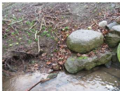
Erosion i NØ-skråning.
